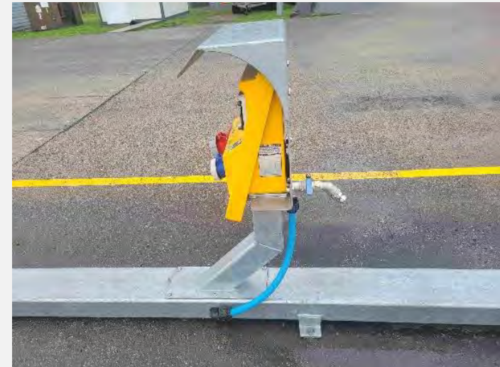
Rear of new power and water pedestals showing water tap for berthed vessels
