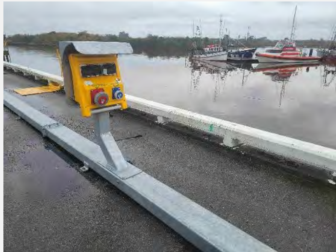
New power and water pedestals (note power and water now moved onto deck of wharf and protected under a steel flange)
