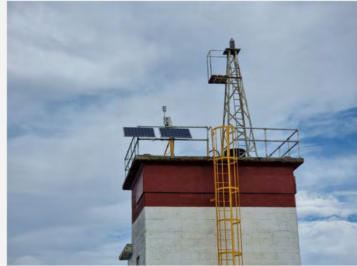
New height access (ladder) system upgrade for bar monitoring system
