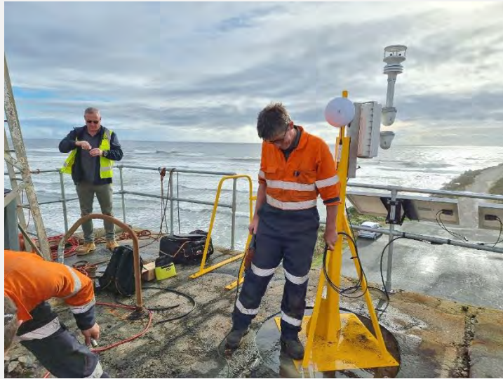
New monitoring (weather, swell, camera) system at Buller River bar
