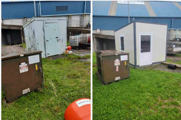
New electrical switch room as part of major power upgrade (old 'room' left; new facility on right)
