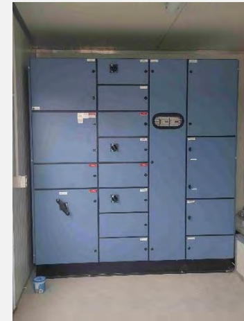
Upgraded electrical switchboard
