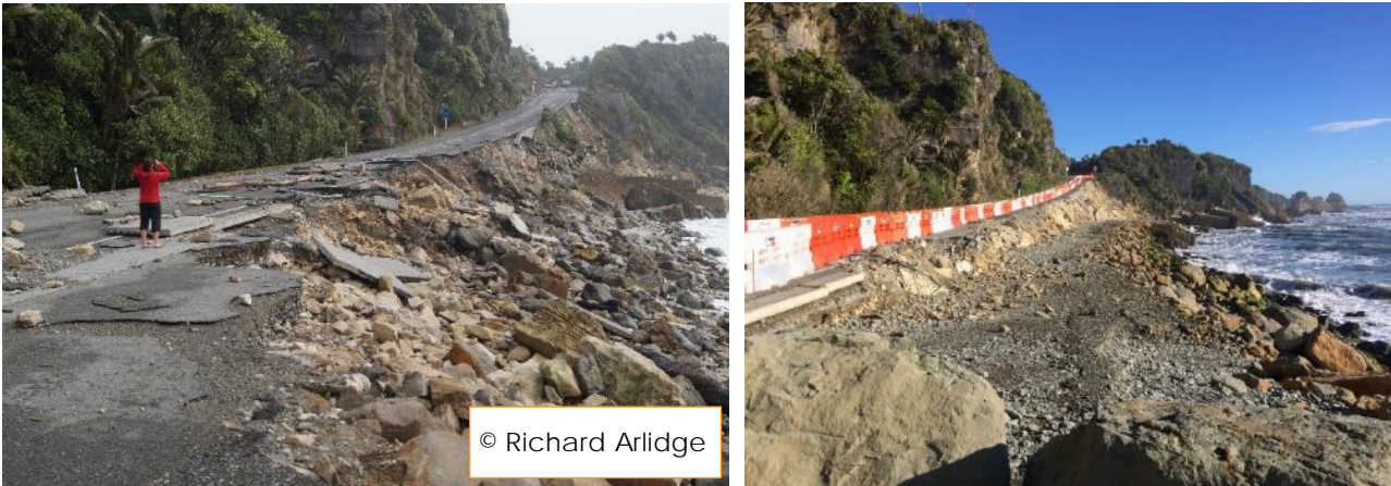
Figure 3-3: SH6 between Dolomite Point and Punakaiki Village shown immediately after ex-cyclone Fehi (left) and as at June 2018 (right)
