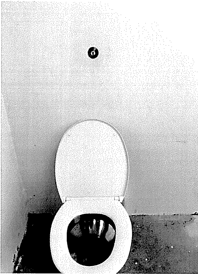
Toilet flush buttons need replacing
