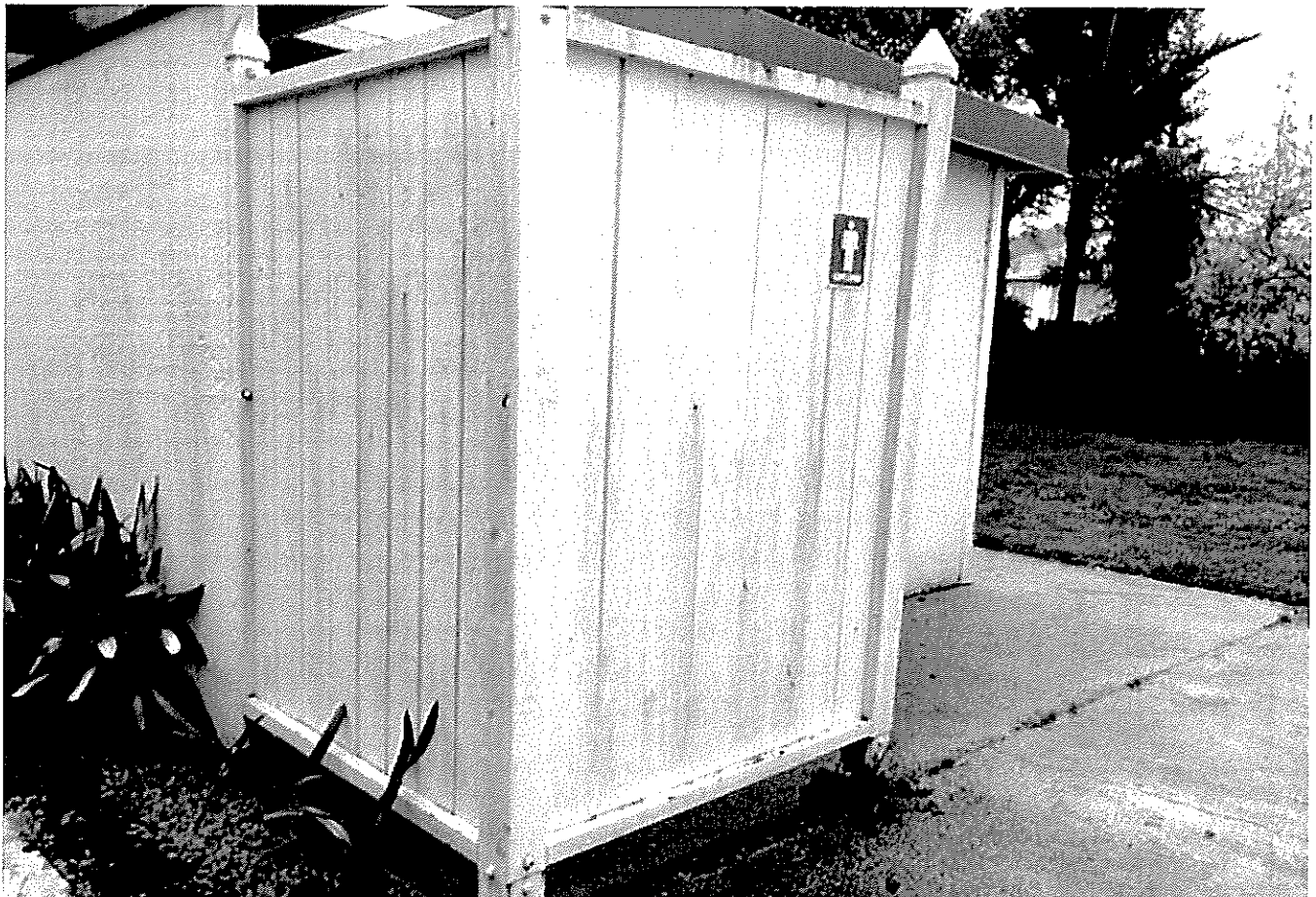
Exterior of entrance to men's toilet needs water blasting
